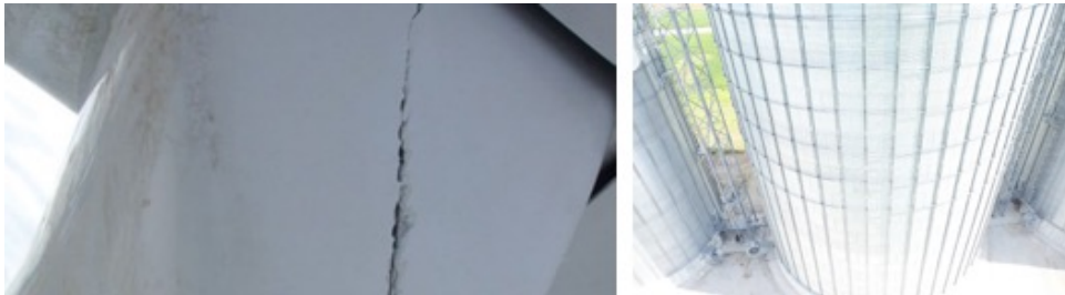
Fig. 9. Sample UAV images of civil infrastructure systems: with cracks (left) and without cracks (right) (Source: InfraDrone LLC)
